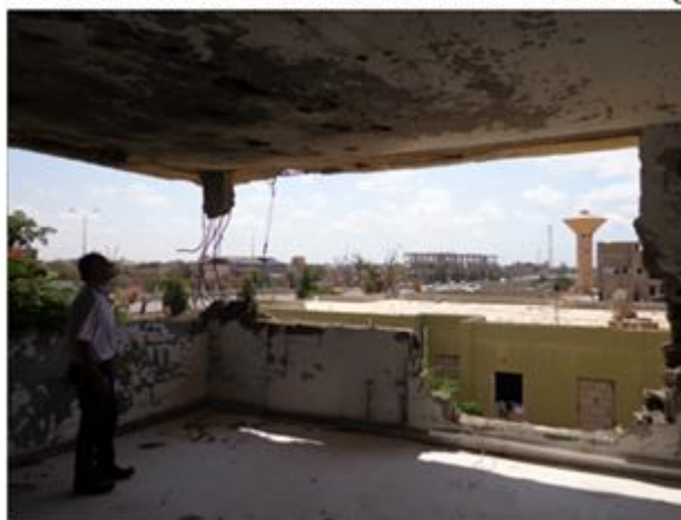
Photo 1.3 Failed column and deflected slab
