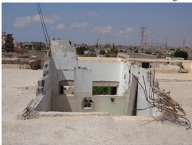
Photo 1.4 Collapsed stair case
