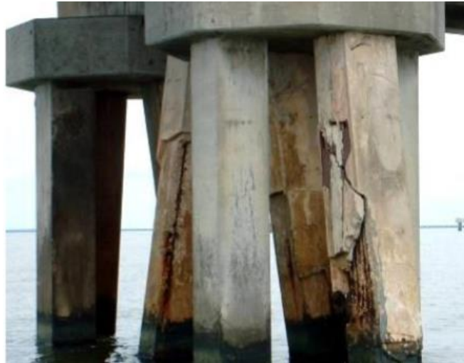
Figure 1 Corrosion in precast prestressed concrete piles [4].
