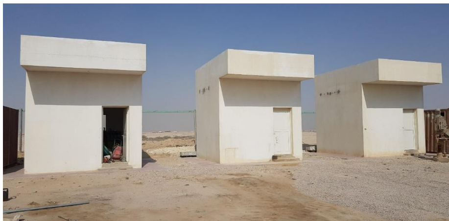
Figure 16 Trial buildings, 4 years after construction: control (100%) gabbro on left; 50% Wadi gravel in centre; 100% Wadi gravel on right.
