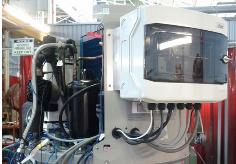
Figure 1 Controller unit mounted inside an enclosure to avoid an ignition source.
