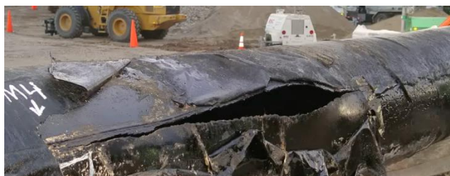
Figure 2 Hydrogen induced cracking of pipeline (Wikipedia).
