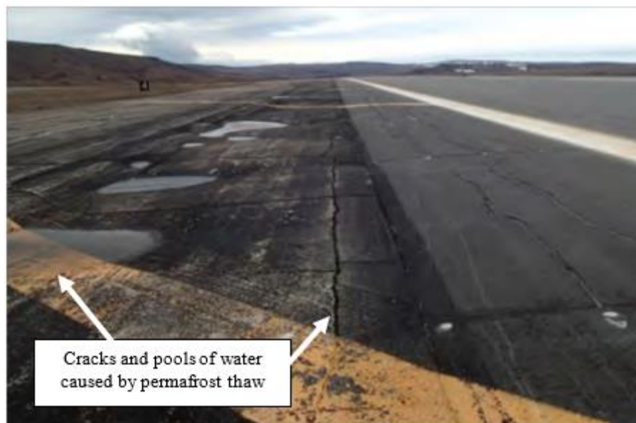
Figure 3 Cracked runways at Thule (Pituffik) AFB, Greenland, from permafrost thaw and refreezing (adapted from [6, 43]) The cracking exemplifies thaw-induced differential settlement at an operational U.S. installation and motivates the foundation and passive-cooling strategies examined in Section 4.
