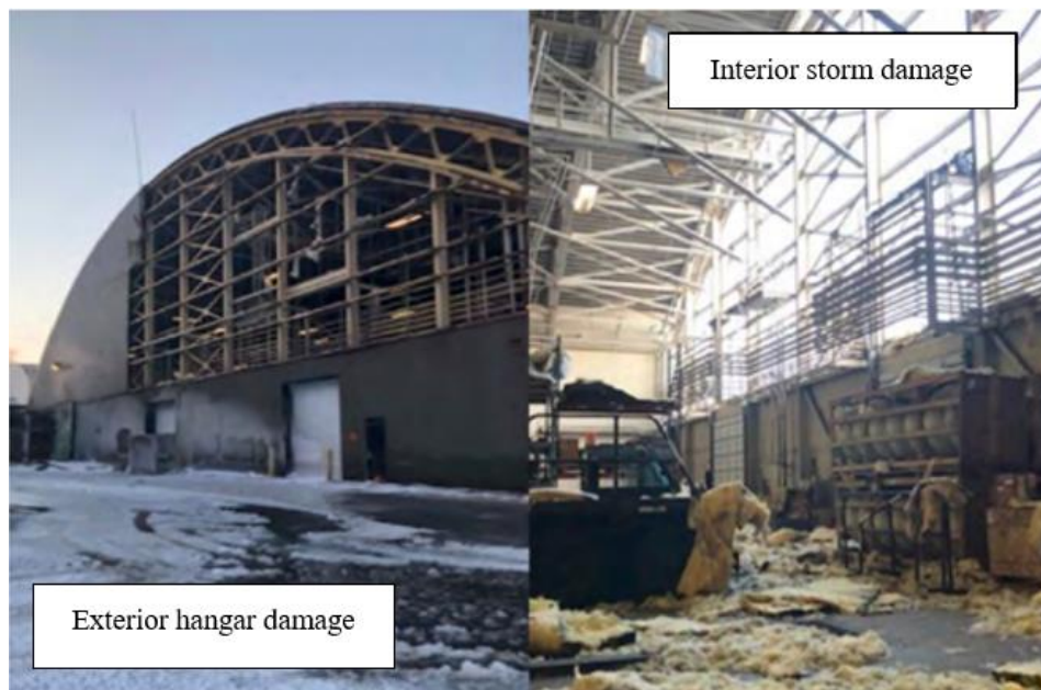
Figure 4 Storm damage to hangars at Eareckson Air Station, Alaska (adapted from [6, 43]). The damage illustrates how compound coastal stressors-storm surge acting on already-exposed infrastructure-translate directly into lost operational capacity.
